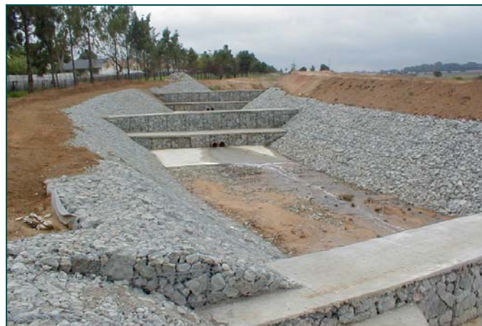
Gabion weirs to dissipate energy and protect the bed canal
