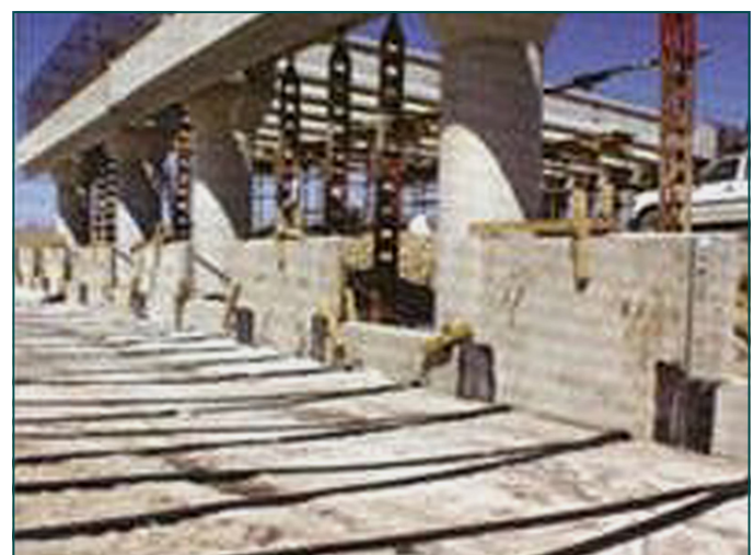
A ParaWeb installation at Maccaferri SA's first MacForce project in South Africa for the construction of abutments on a Western Cape bridge.
