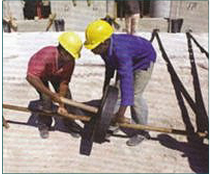
Looping the ParaWeb soil reinforcement under a temporary stay, which assists in tensioning the strip.
