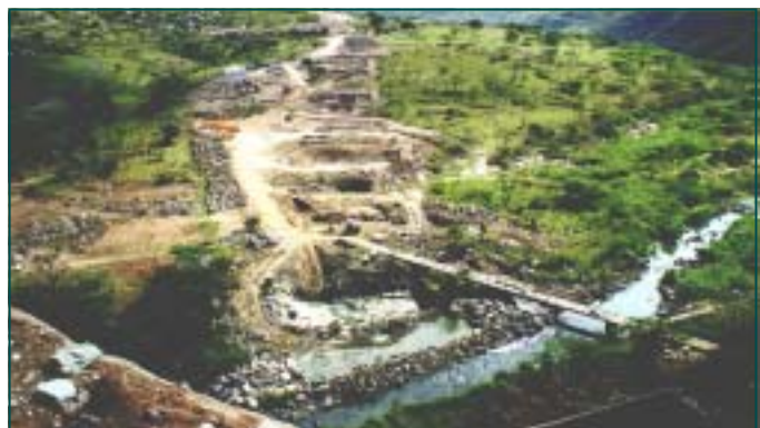
A view across the valley where the Mgeni Viaduct will be constructed over the Umgeni River in Kaw-Mashu.
