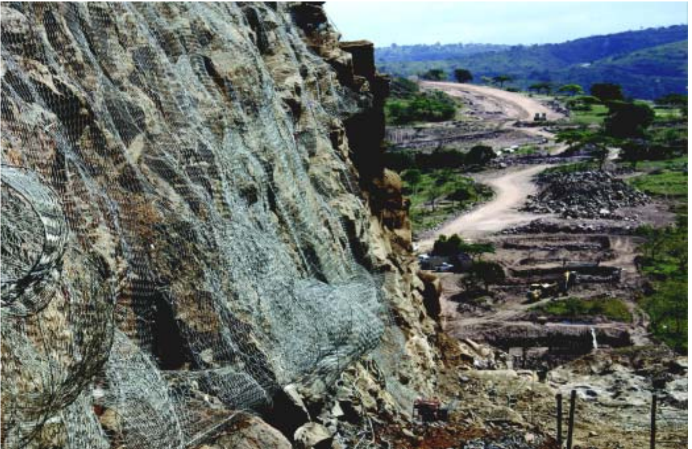
A view of the route for the Mgeni Viaduct with SteelGrid MO installation in progress.
