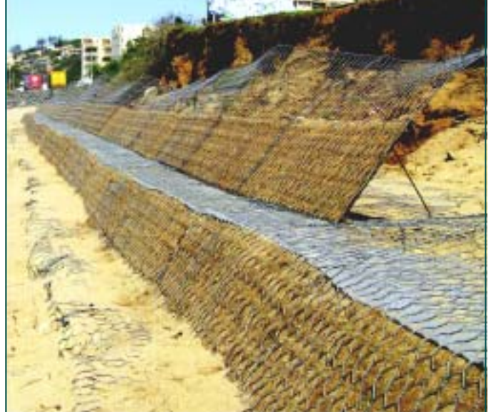
Green Terramesh panels lined with Maccaferri’s BioMac biodegradable erosion control blanket. The Terramesh System used to construct the Umdlotti wave dissipation structure is concealed below the sand. The area behind will be backfilled to form the final slope profile.
