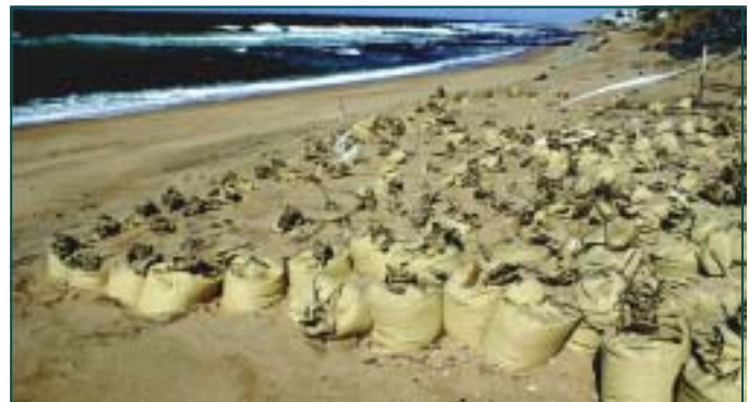
Sandbags ready for use in constructing the Terramesh System units. Their adoption instead of using rocks is a first time application in KZN.
