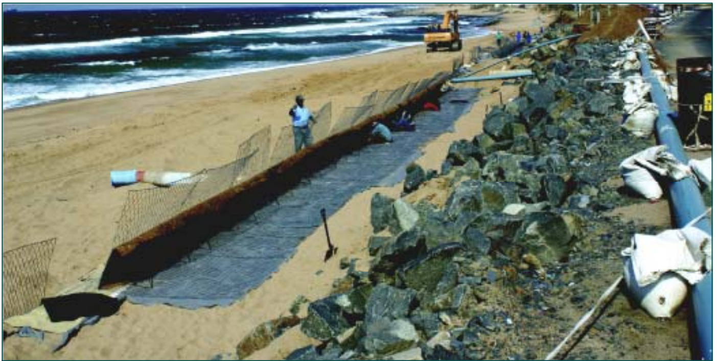
Green Terramesh construction in progress. On the right are rocks that were temporarily dumped to protect the roadway to prevent it from being undermined following severe storm damage.
